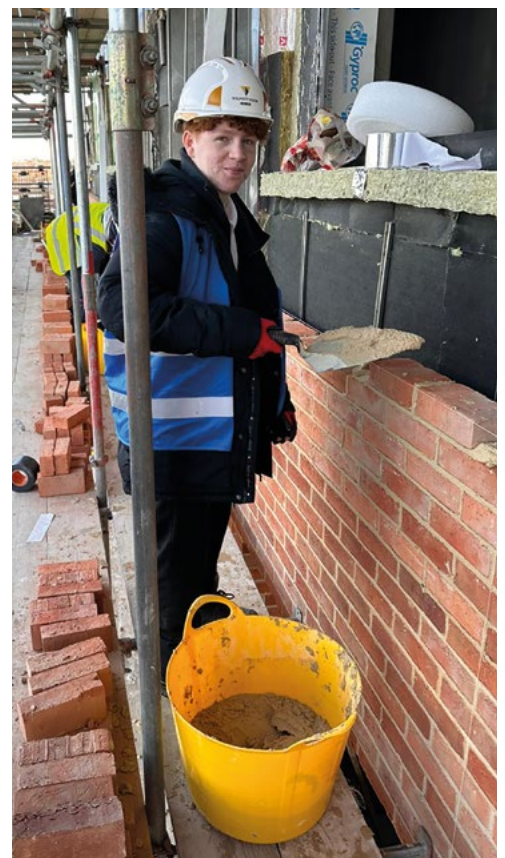
Zack, a year nine student at Dagenham Park School. Trying out bricklaying on Wheeler's Court in the Gascoigne Neighbourhood.
